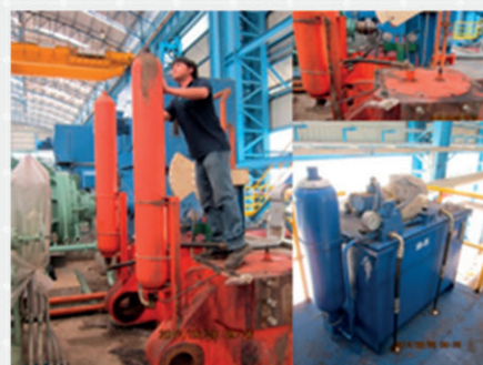
Accumulator & Power unit
